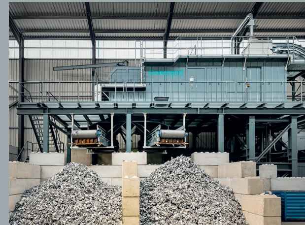
Recycling of recyclable materials with high throughput, © cleansort GmbH.
